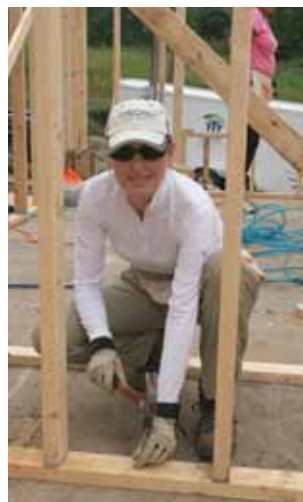
Help an O.C. family in need during our next Habitat for Humanity build in Fullerton.
