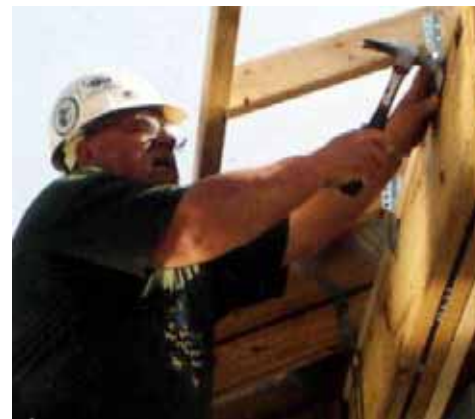
Bruce finishes off the porch roof of a house in Biloxi, Mississippi, not long after Hurricane Katrina.
